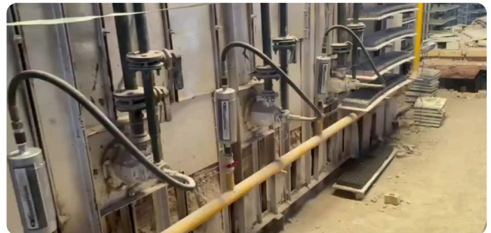
Modules on the gas feeds along the kiln wall. Niveda Green site photo and video still, 2026.
