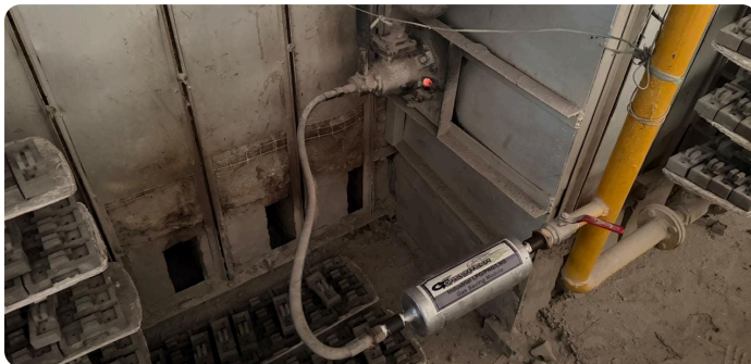
A Greentech Industrial Gas Saving Module on the PNG feed to one of the kiln's burners, trays of fuse bases alongside.
